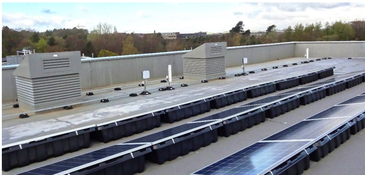
Solar powered ventilation units and solar PV array, the Lyell Building, Edinburgh Campus
