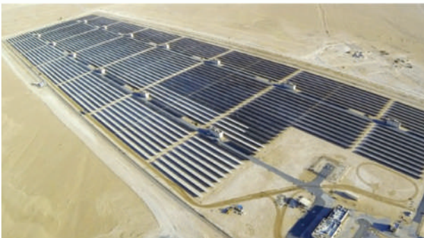
Aerial view of Mohammed Bin Rashid Al Maktoum Solar Park (image source: Day of Dubai, 2016)
